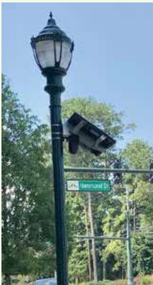
Solar & Existing Pole
