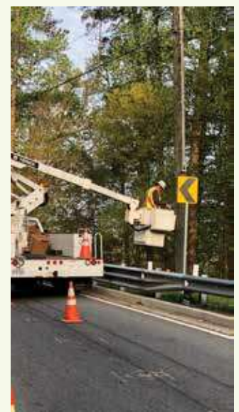
Electric & Existing Pole
